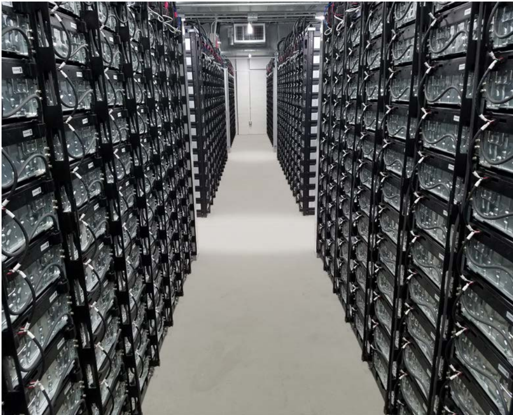
Figure 7. 20 MW / 80 MWh ESS in California with planned augmentation and flexible warranty.
